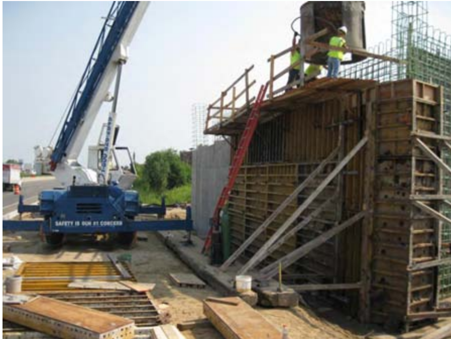
Concrete pour of the south half of the east abutment stem wall. The completed and stripped north half can also be seen in the background.
