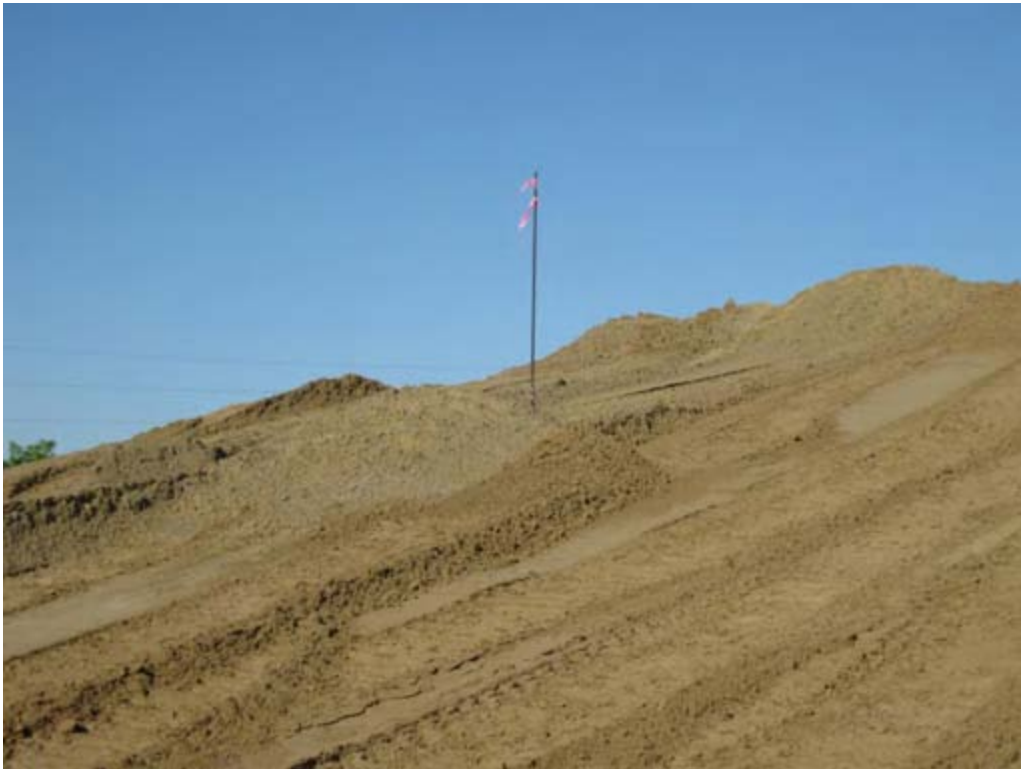
Settlement plates placed below the embankment material are attached to a series of poles (pictured) that are used by Washington County surveyors to track settlement
