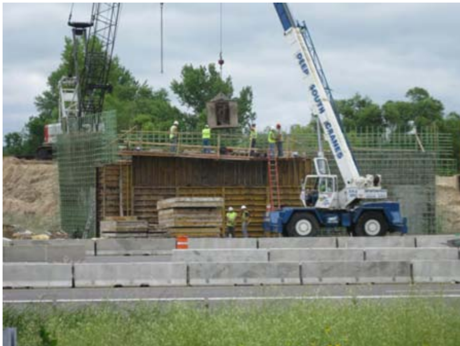
Workers pouring concrete for the north half of the east abutment stem wall
