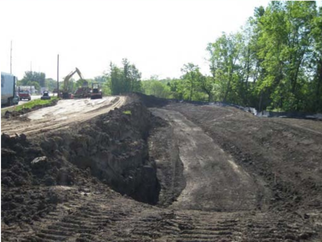
Excavation work on the east infiltration basin located just south of CR 83 at 15 th Street
