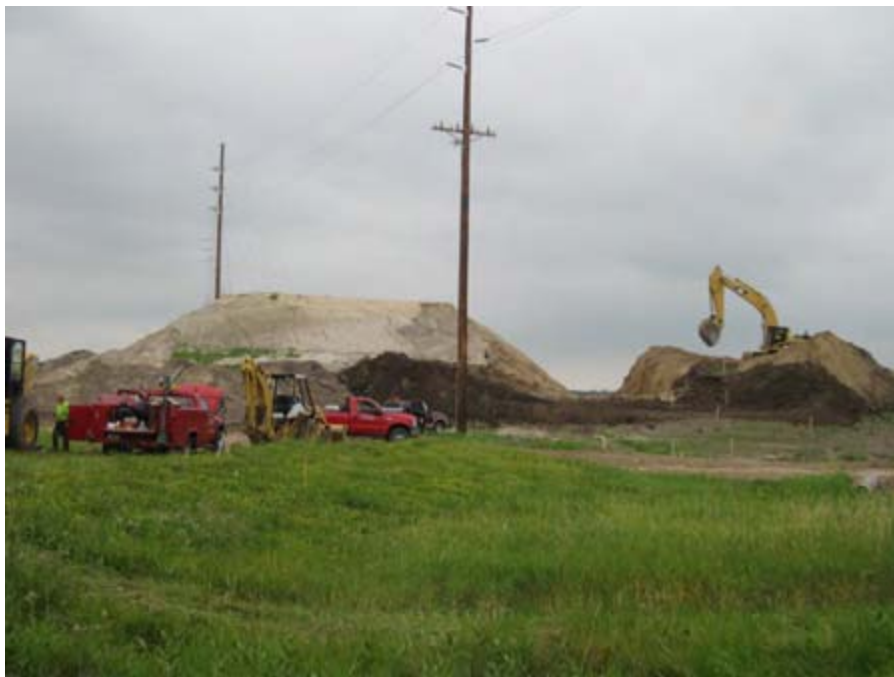
Excavation through the west embankment for placement of a storm sewer culvert.
