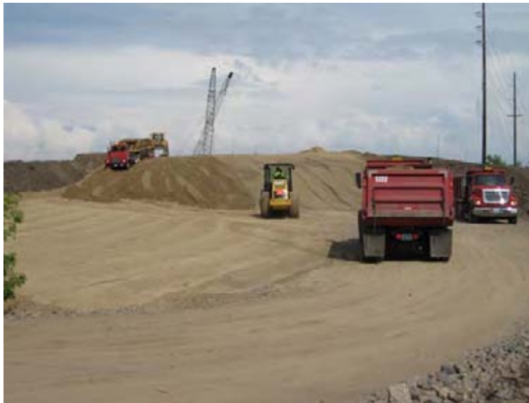
Forest Lake Contracting hauling granular material for the embankment west of I-35
