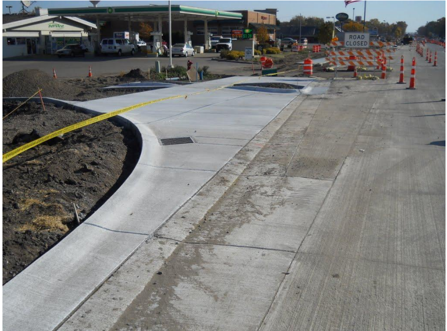
A look at a newly constructed driveway apron on the east side of the project
