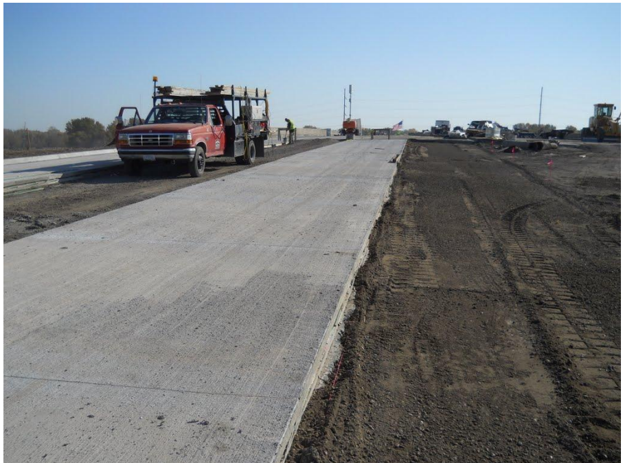
Concrete paving in the interchange area on the west side of the project
